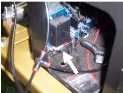
Figure 8.5 Remote control fuse location
